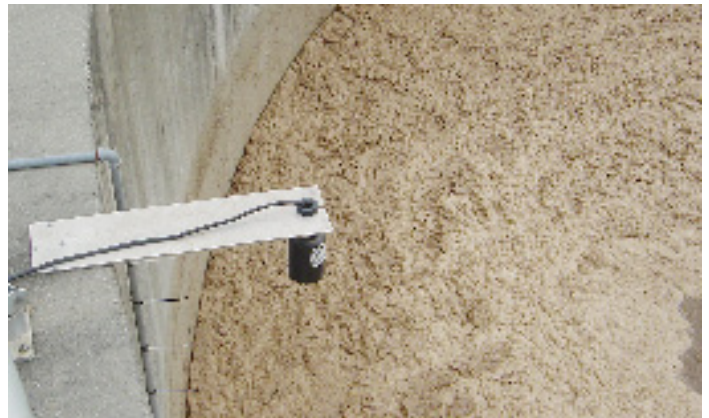
K10C ultrasonic transducer installed at a wastewater facility.
