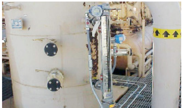
KM26 magnetic level gauge installed on a separator
