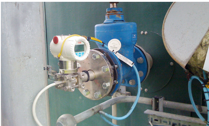
266T differential pressure transmitter installed for a digester level application
