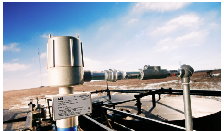
LevelMaster installed on oil tank batteries
