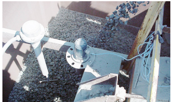
LM80 laser installed on ore surge bin
