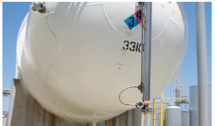
KM26/AT200 installed on a chemical storage tank
